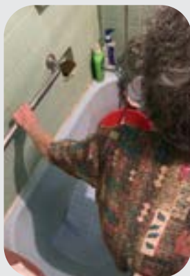
Installation of handrail and non-slip mat in bathroom to reduce fall risk
